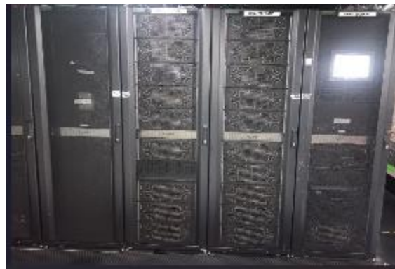
100% - Modular UPS (Efficiency - 99%)
